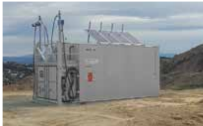
Solar Tank for Farming Client New Zealand
