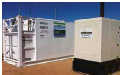
Back-up for Power Generation Australia
