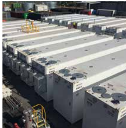
WESTERN TURNER PROJECT - 11 x Classic Tanks Diesel
