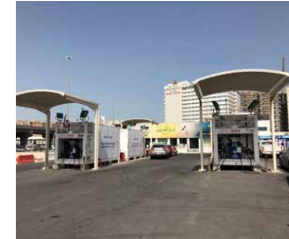
MODULAR FUEL STATION, QATAR
